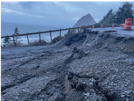
A 200-yard section damaged due to landslide Credit: By OregonDOT CC BY 2.0
