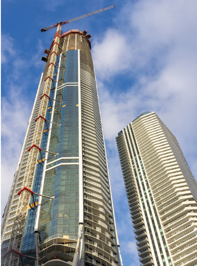
Construction of SkyTower next to Prestige at Pinnacle One Yonge in Toronto, ON "Pinnacle One Yonge Construction, November 16 2025 (06)" by Dillon Payne is licensed under CC BY-SA 4.0
