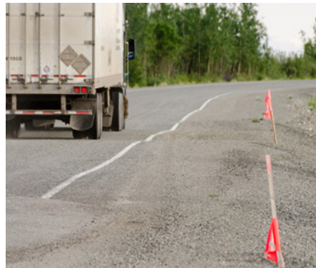
Klondike Highway is in the extensive discontinuous permafrost zone Highway surface distortion on the Alaska Highway Source (both photos): Yukon.ca Driving on permafrost-affected roads © Government of Yukon 2026
