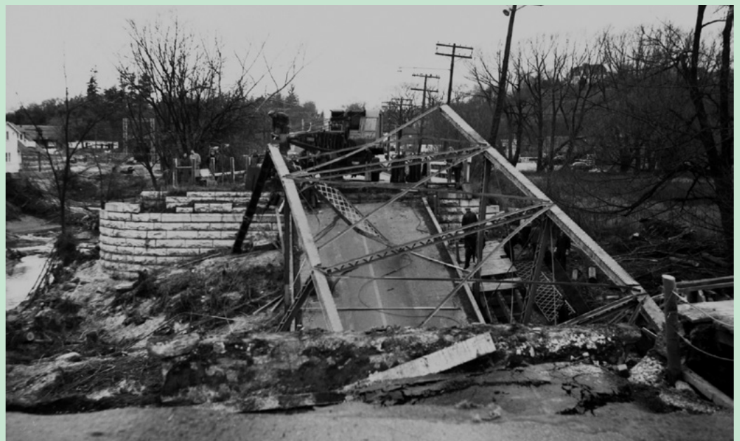
Don R. (West Don R.) looking north across Yonge St. bridge-Hurricane Hazel 1954 Courtesy of Toronto Public Library- Public Doman
